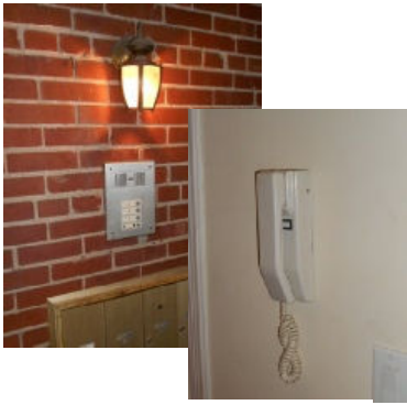
Secure lobby door with intercom and electric door strike system.
